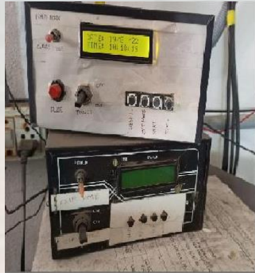
Automatic Overhead Tank Water Control
